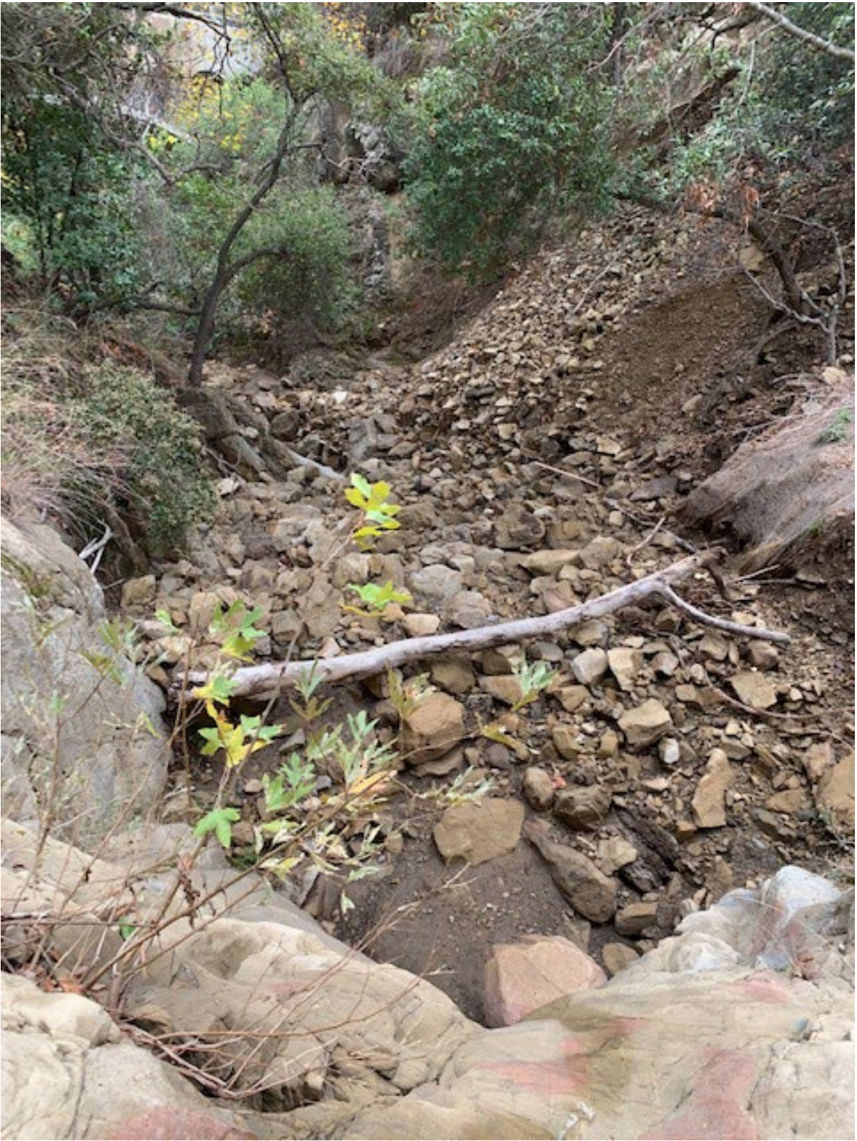
Figure 3.13. Rockfall reaching Mission Creek's channel. Rockfall originated from canyon slope exposed along Tunnel trail (see Figure 3.11). Coordinates: 34° 28.963' N; 119° 42.426' W.
