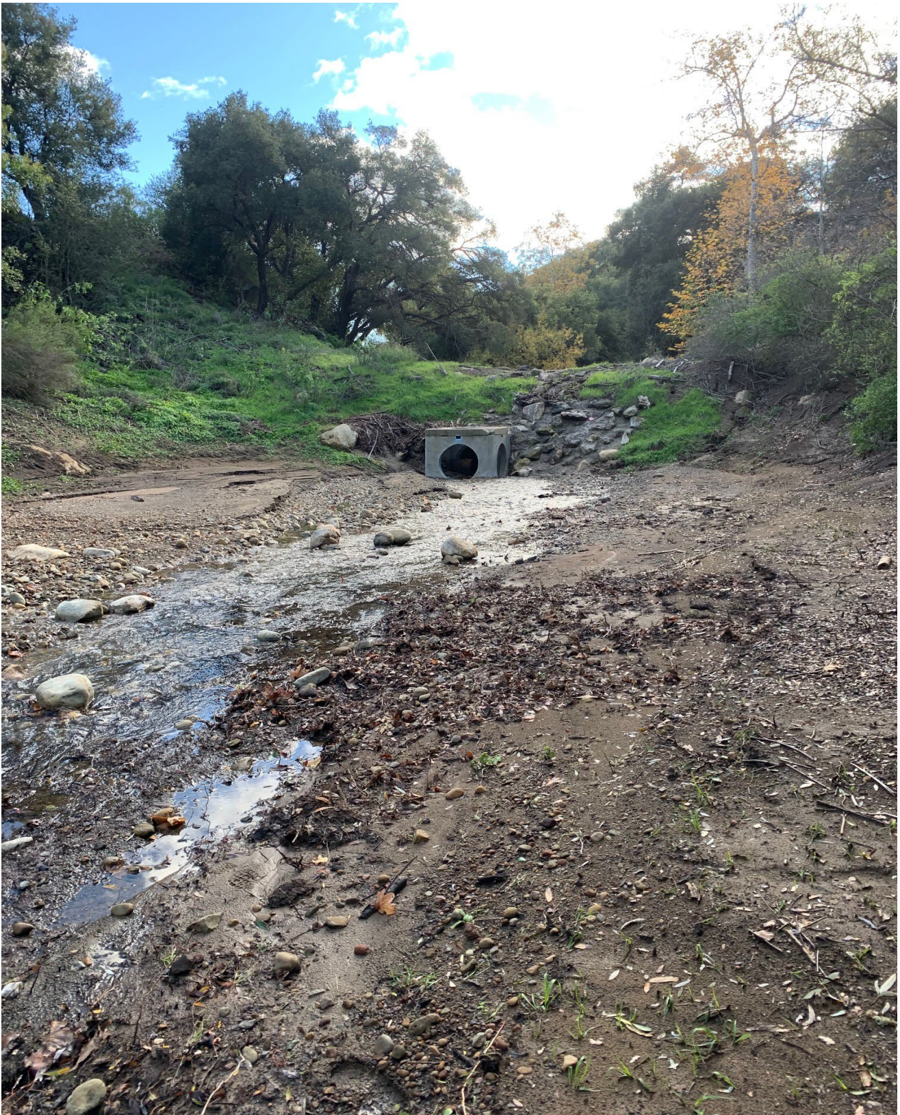
Figure 3.4. Photograph of the debris basin in Mission Creek looking downstream. A concrete intake structure was built to reduce obstructions by large woody debris inside the culvert.
