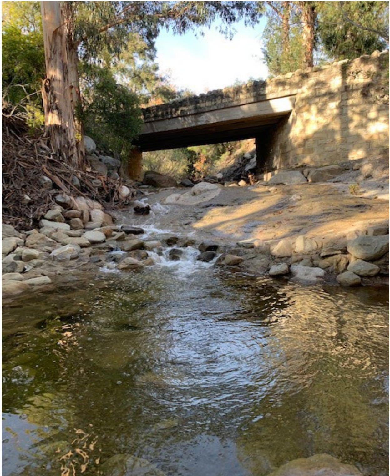
Figure 3.7. Photo of Mission Canyon Road over Mission Creek, viewing north or in the upstream direction (coordinates: 34° 27.124' N; 119° 42.564' W).
