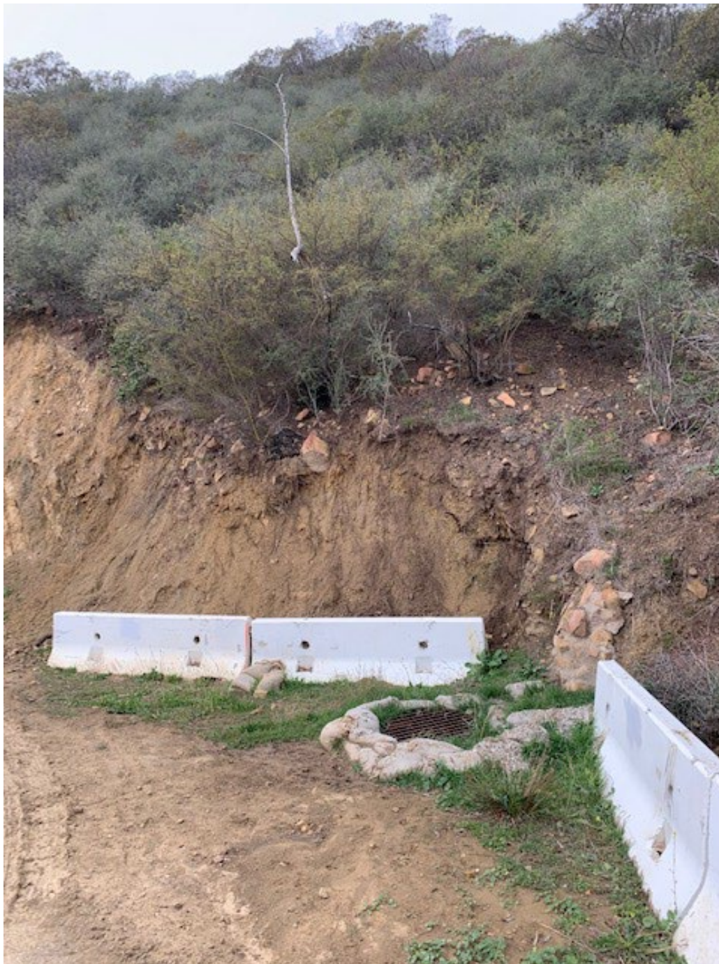
Figure 3.14. Photo of the right side of Tunnel trail viewing south. The eroding slope and manhole at the base of the slope convey moves sediment laden runoff through a culvert towards Mission Creek located towards the left of the trail. Dense chamise chaparral covers the mountain side.
