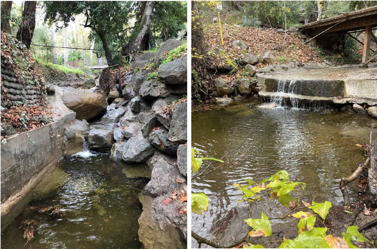
Figure 4.1.23. Fish passage impediment along a channelized section of the creek (left). The scour depth of the channel bed sediments at its downstream end is ~1.5 m creating a ~3 m jump to the modified channel above (left). A pool formed below a concrete slab at a bridge crossing creates a ~1 m high jump (right). Photographs taken on December 16, 2021, during low flow conditions.
