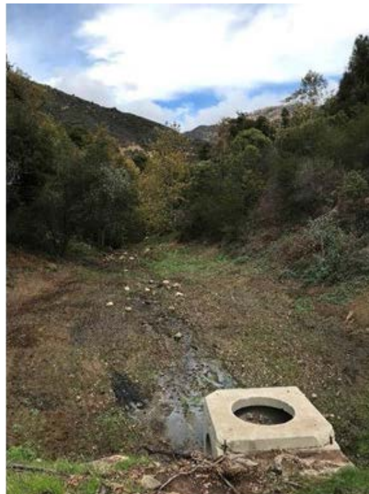
Figure 4.1.10. (a). The plunge pool on the downstream side of the debris dam is ~2m deep, and the top of the debris dam is ~6.5 m above the water surface. Photo taken on December 28, 2021. (b). View looking upstream for ~ 65 m from the debris dam. Photo taken on December 9, 2021.
