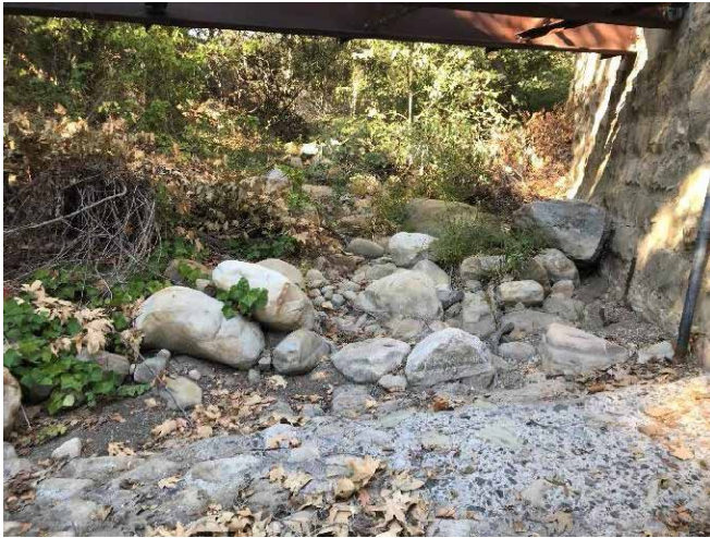
Sediment deposition upstream of the Mission Canyon Rd. bridge extends for ~20 m upstream. Photo taken on December 12, 2021 during base flow conditions.
