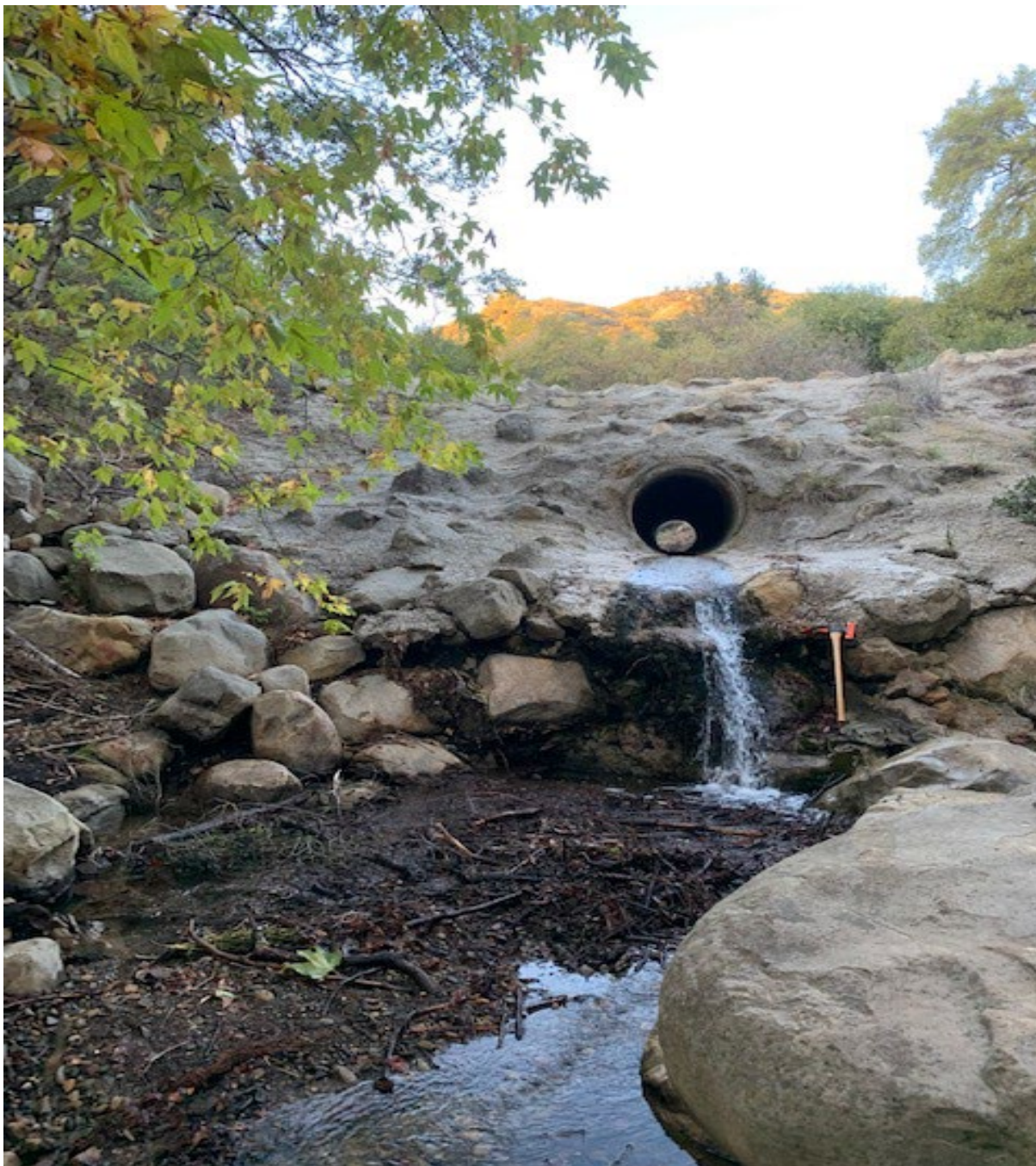
Figure 3.20. Debris dam in Rattlesnake Creek. Photo viewing upstream (coordinates: 34° 27.587' N; 119 41.531' W).
