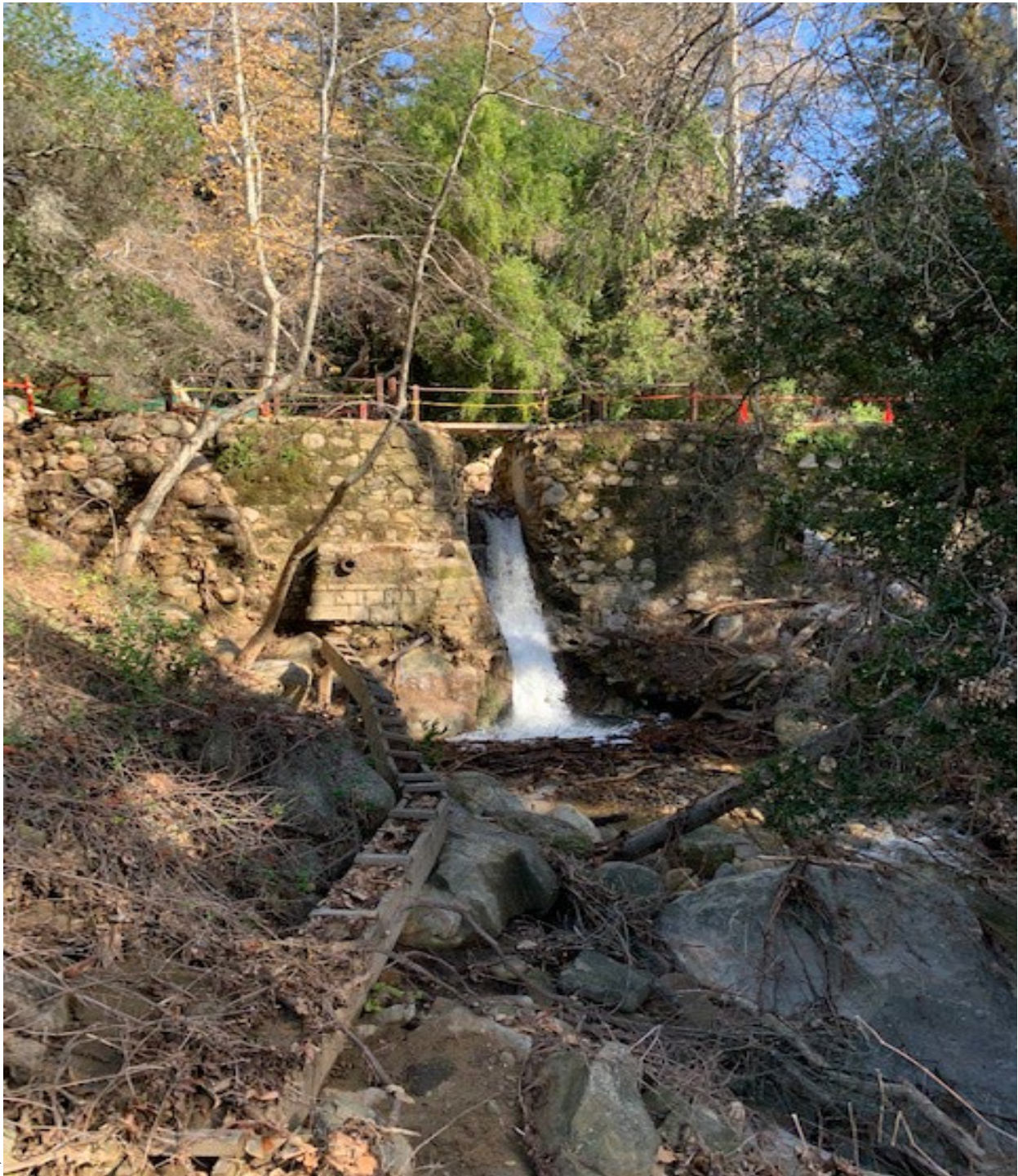
Figure 3.1. Photo of Mission Dam viewed in the upstream direction. A wooden portion of the ancient aqueduct is seen on the left side of the photo (the right bank of the stream). This photo was taken after the heavy rains in January 2023. The storms of January 2023 transported large amounts of woody debris downstream from the upper Mission Creek watershed, causing the dam to be over-topped, and eroding portions of the west abutment. The unreinforced boulder and brick dam may be subject to potential catastrophic failure in future flood events. Coordinates: 34° 27.521' N; 119° 42.606', elevation 733 feet above mean sea level.
