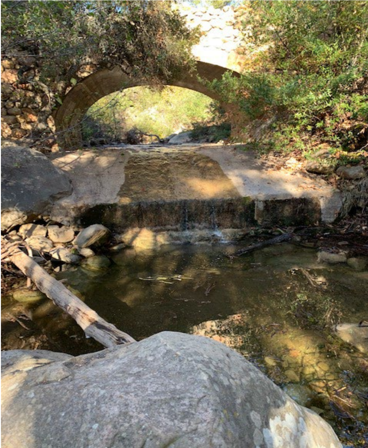
Figure 3.17. Photo viewing in the upstream direction at Las Canoas Road bridge over Rattlesnake Creek (coordinates: 34° 27.441' N; 119° 41.525'W).
