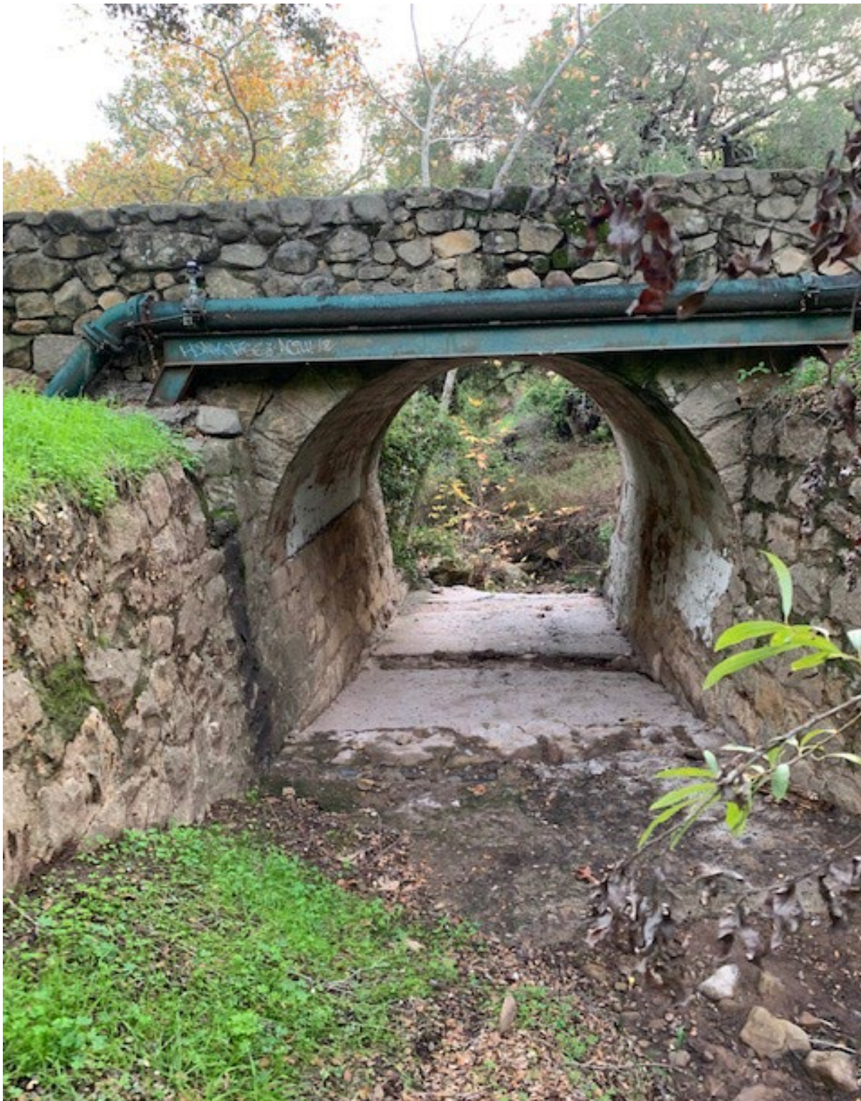
Figure 3.25. Bridge on Las Canoas Road over a tributary stream to Rattlesnake Creek. Photograph looking downstream (coordinates: 34° 27.124' N; 119° 42.564' W).
