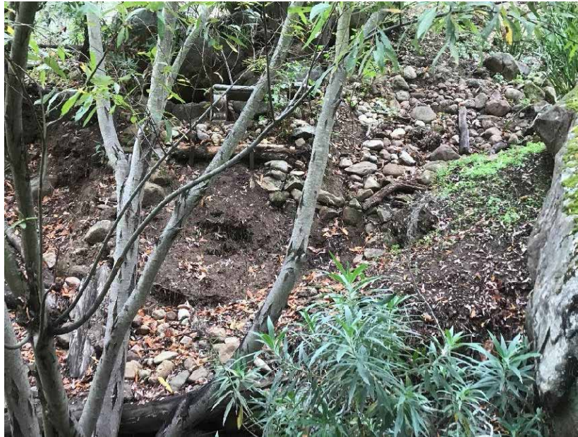
Figure 4.1.9: Construction of streamside bench and private trail upstream of Mission Dam. Small construction projects by homeowners intrude into the riparian and stream environment and increase erosion of fine sediment into the stream channel. Photo taken on December 9, 2021.
