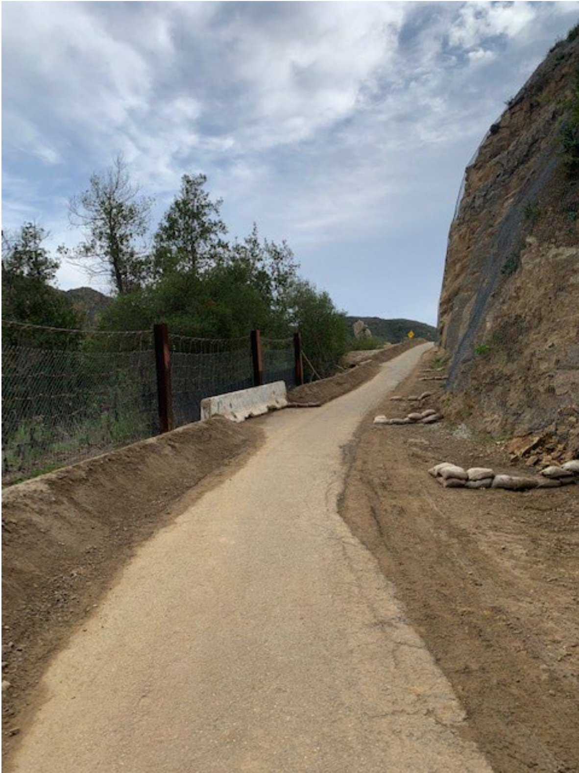
Figure 3.12. Photo of remedial measures taken to contain rockfalls into Mission Creek: metal screens, metal fences, berm, and K-shaped concrete wall. Photo looking south along Tunnel trail, uphill from the right bank of Mission Creek. Coordinates: 34° 28.963' N; 119° 42.426' W.
