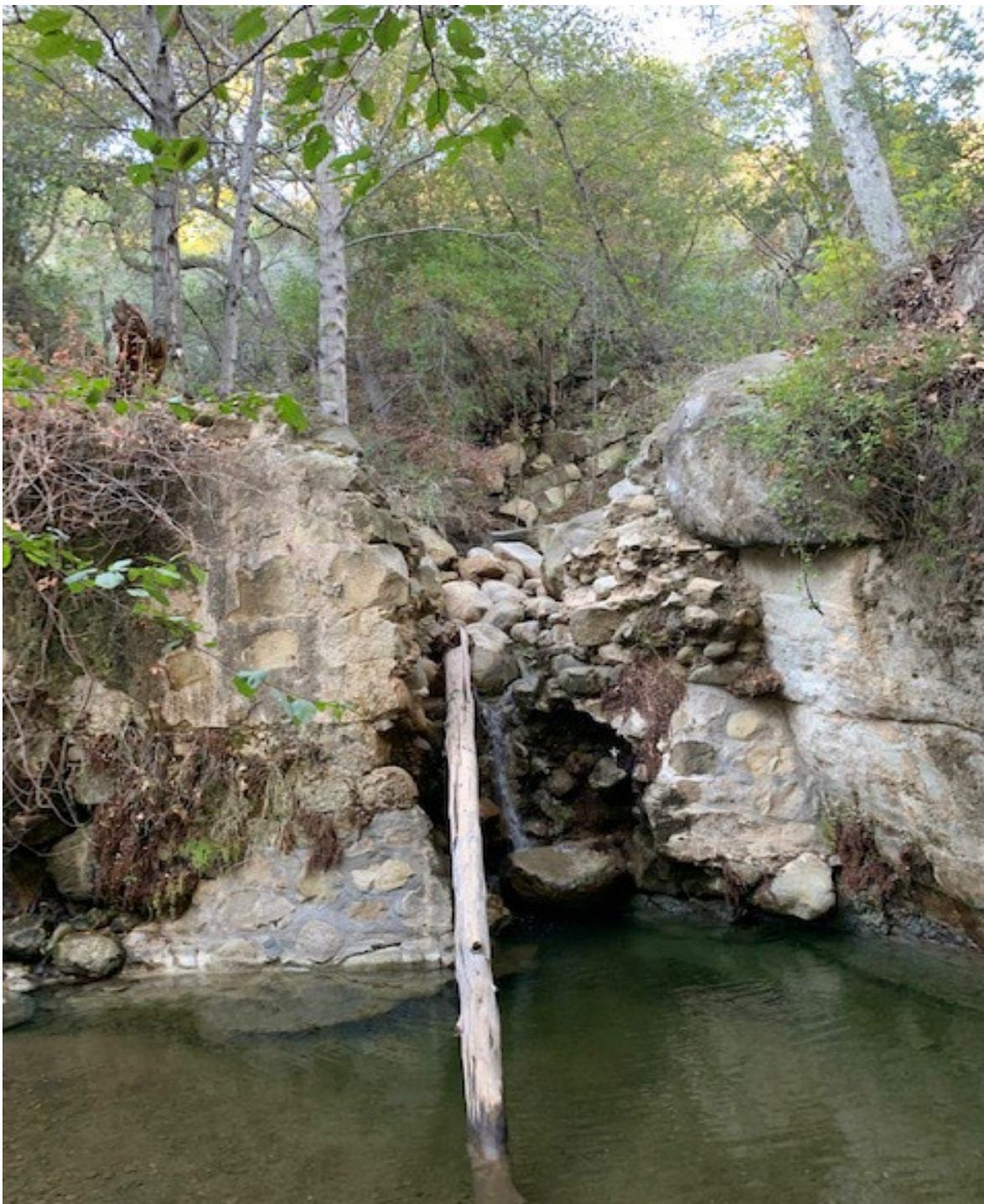
Figure 3.19. Masonry dam in Rattlesnake Creek, partly collapsed (coordinates: 34° 27.762' N; 119° 41.456' W). Photo viewing upstream.
